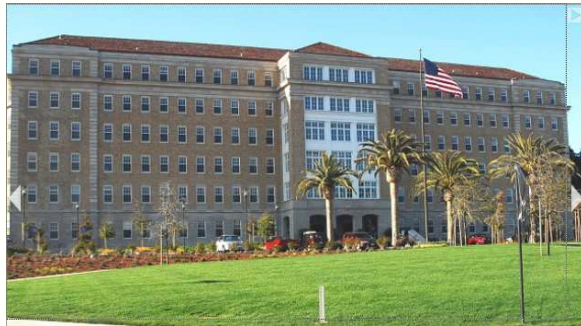
Replacing limestone cladding panels with FRP panels on the Public Health Services Hospital in San Francisco's Presidio Park.
